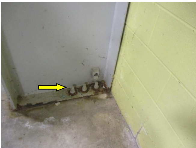
Corrosion noted on the columns.
