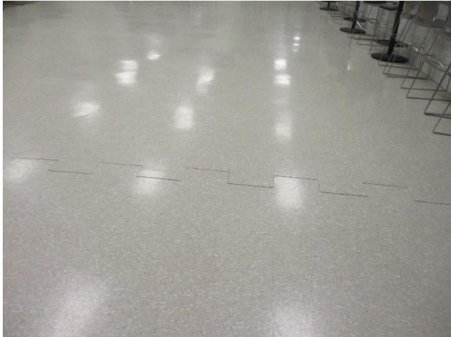
Gapping floor tiles on the mezzanine indicates movement of the subfloor.
