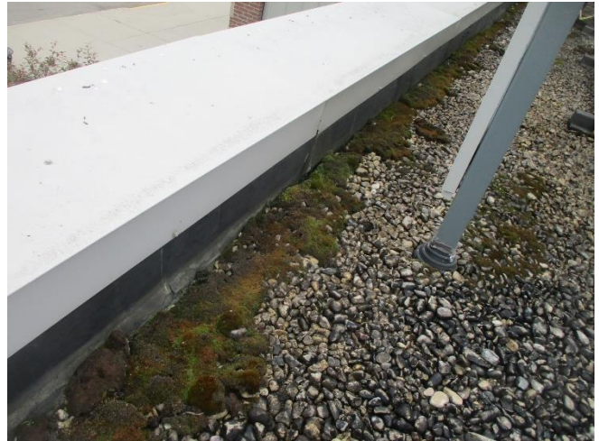
Roof C1.1: Organic growth on the roof.
