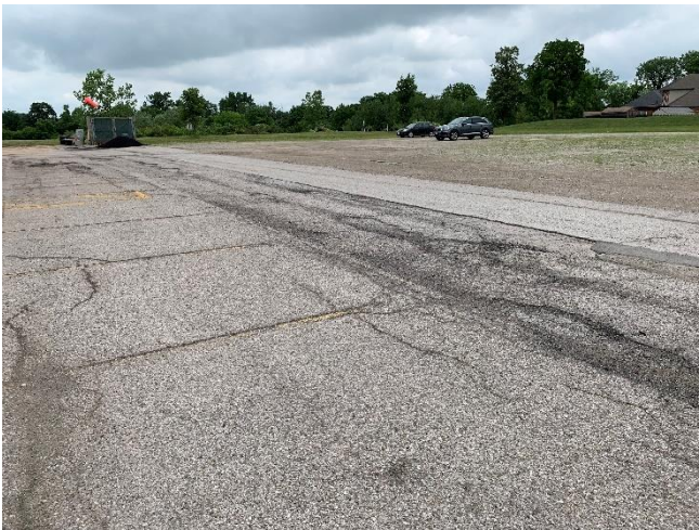
Deteriorated asphalt pavement on the northeast portion of the Site.
