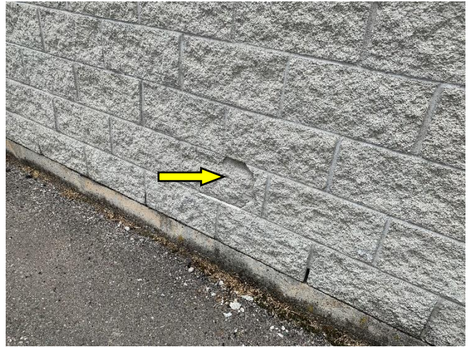
Impact damage noted on the west elevation. .
