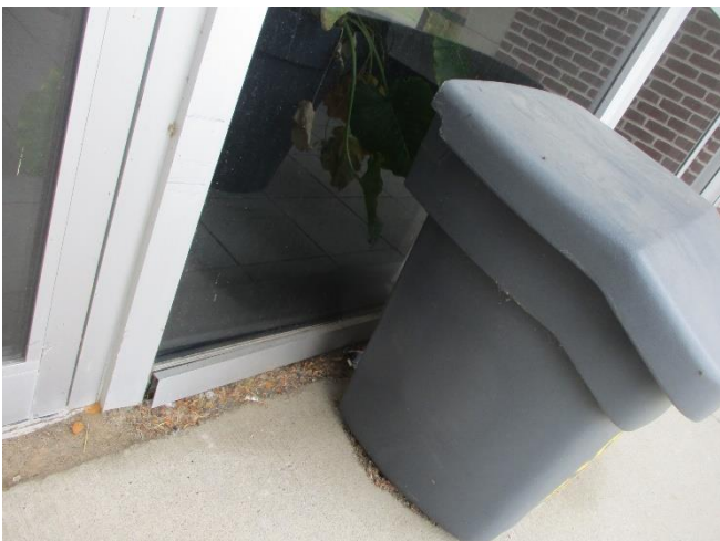
Damaged exterior face of the main door framing.
