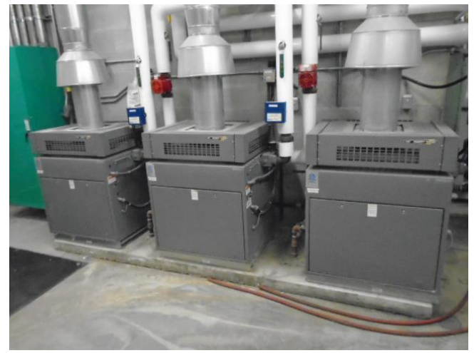
View of domestic water heating boilers.
