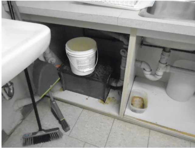
View of grease intereceptor in concession area.
