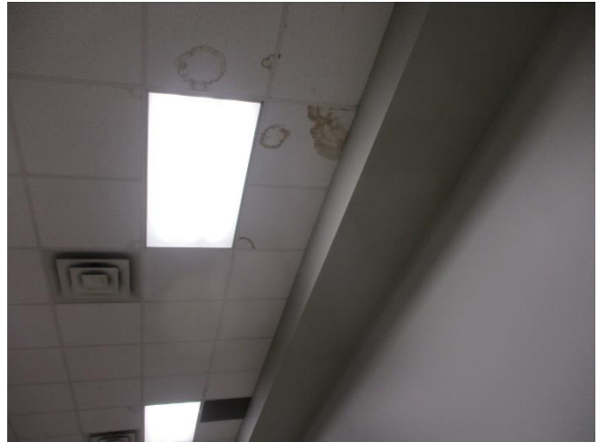
Stained ceiling tiles at the community hall.
