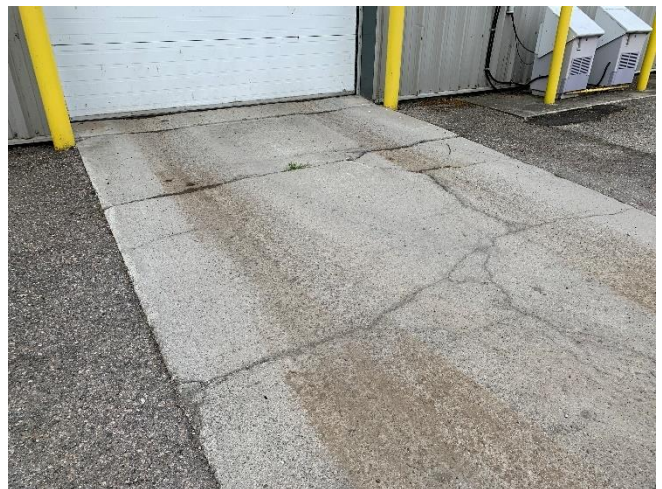
Deteriorated concrete pad adjacent to a drive-in door.
