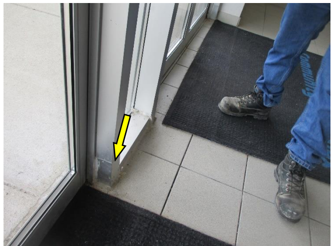
Previously patched main entrance door frame.
