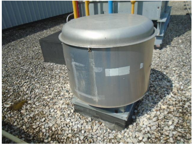
Exhaust fan on refrigeration room roof
