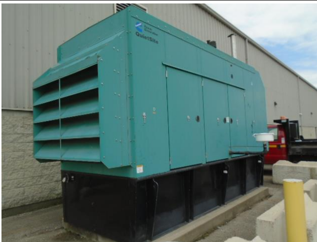
Enclosed generator set.
