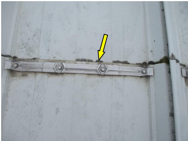
Roof A: Deteriorated sealants at joints.
