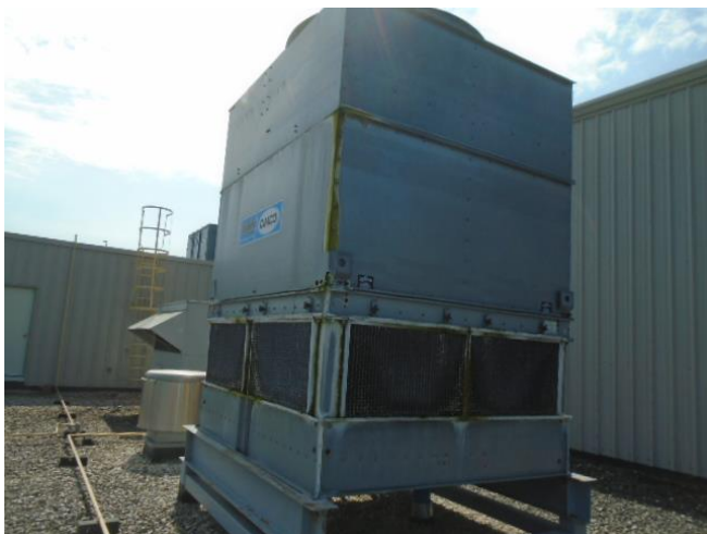
View of cooling tower.
