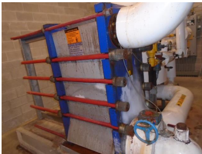
Ammonia heat exchanger.
