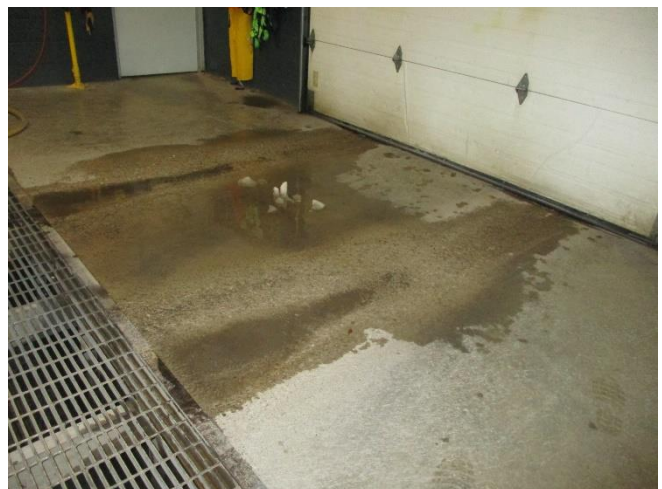
Deteriorated concrete at ice re-surfer room.
