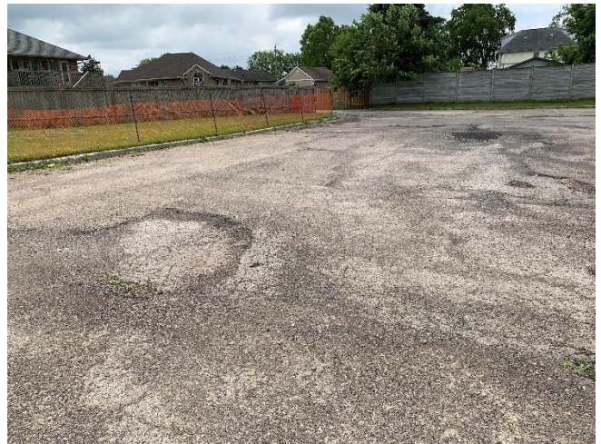
Deteriorated asphalt pavement on the east parking lot of the Site.
