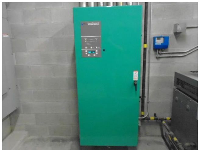
Automatic transfer switch.
