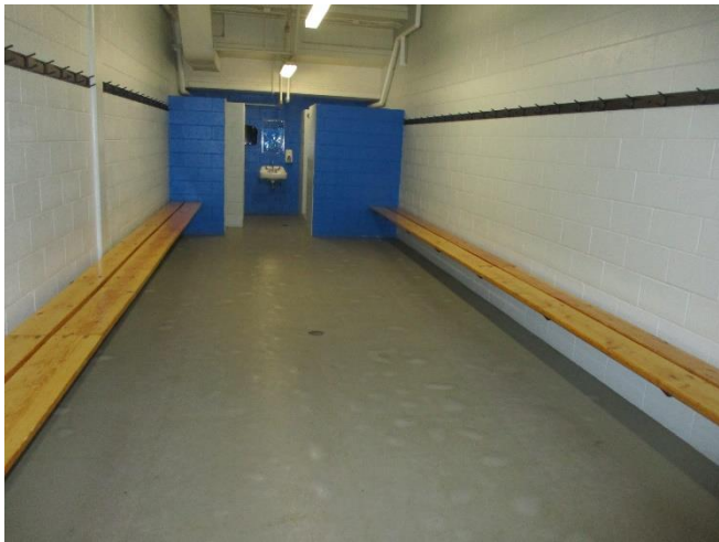
Deteriorated flooring at a change room.
