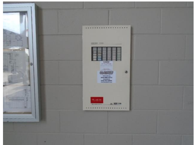
Fire alarm control panel.
