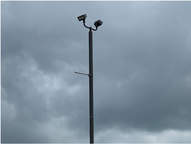
Typical Site lighting feature.
