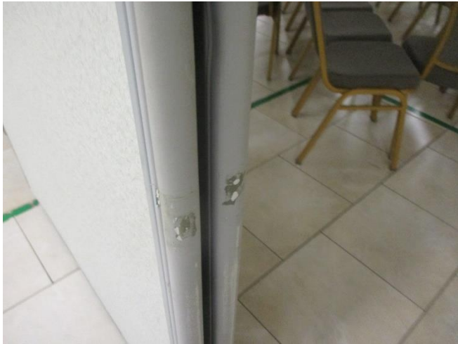
Retractable/folding partition wall at the community hall. .
