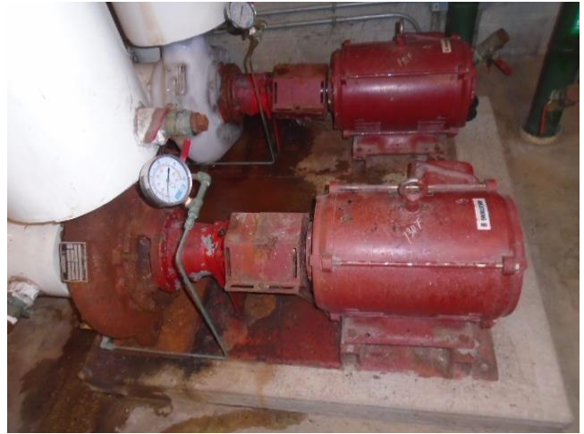
Glycol cooling pumps.
