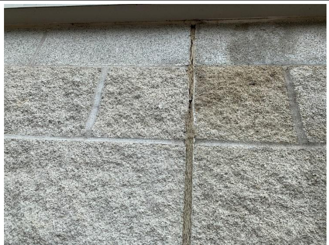
Deteriorated sealant at a control joint.
