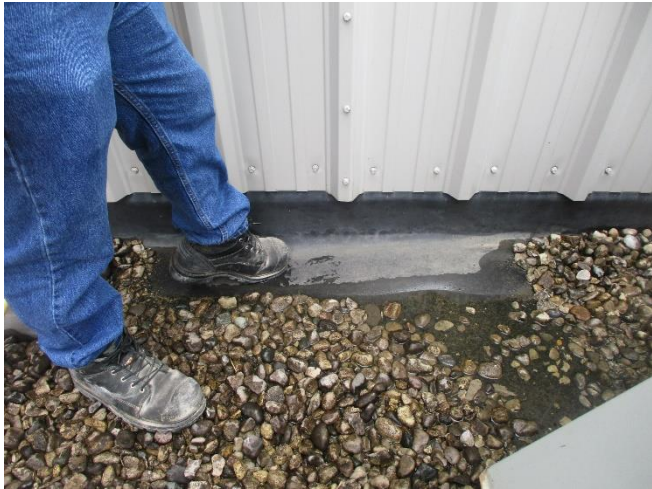
Roof C1.3: Tenting and ponding water.
