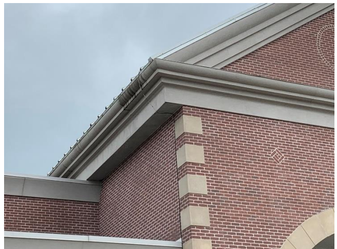
Deteriorated EIFS moulding on the southwest.
