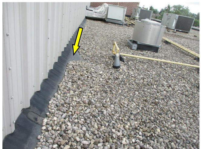
Roof C1.1: Severe tenting at the base of the wall.
