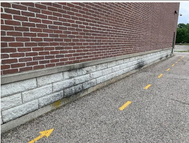
Moisture noted damage on concrete ledge and blocks.
