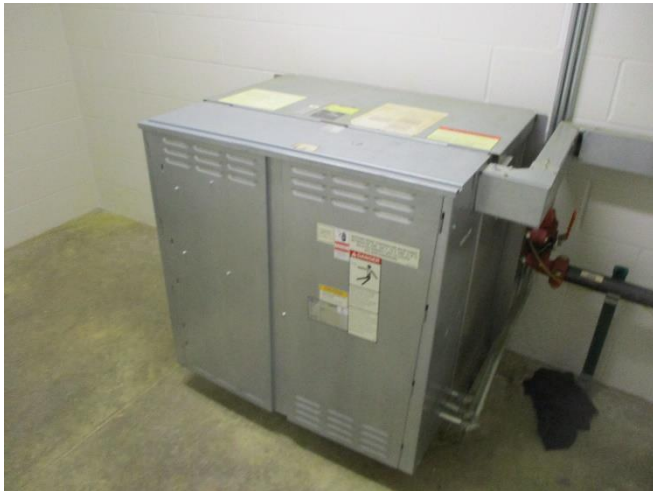
General view of the elevator machine serving the Building.
