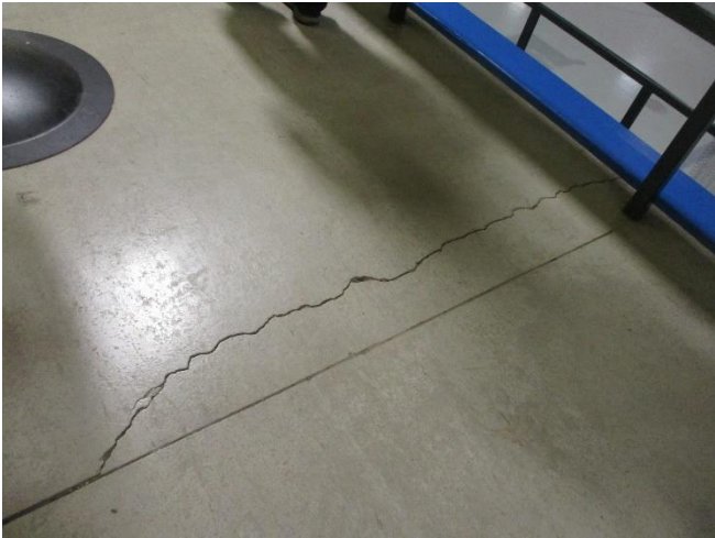
Cracked concrete topping at the seating area.
