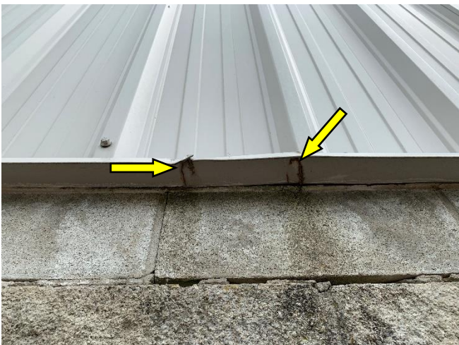
Damaged drip edge at the base of the siding causing water run-off on the masonry.
