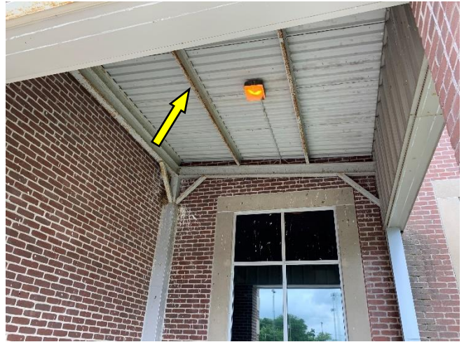
Corroding metal at an exterior soffit.
