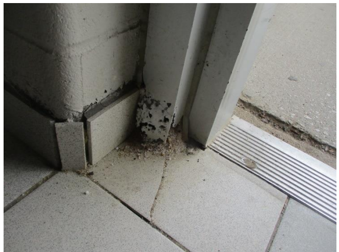
Damaged frame of the main entrance door.
