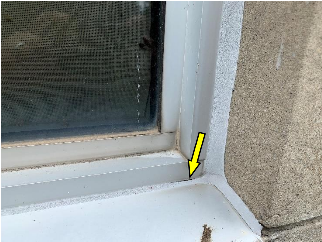
Failing and hardened sealants at a window perimeter.
