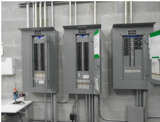
Typical electrical distribution.
