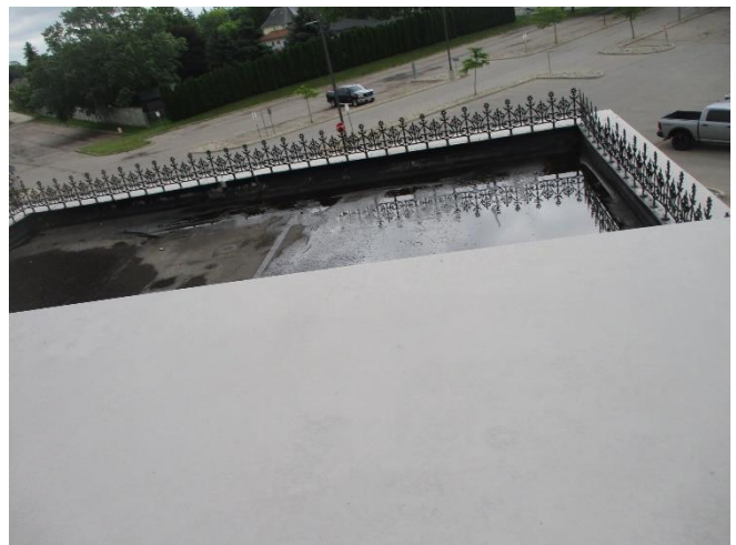
Roof D: Ponding water noted atop the roof.
