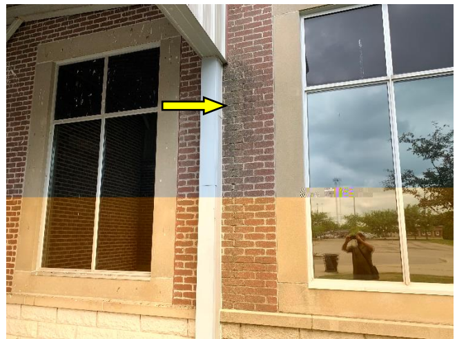
View of moisture damaged brick masonry on the south elevation.
