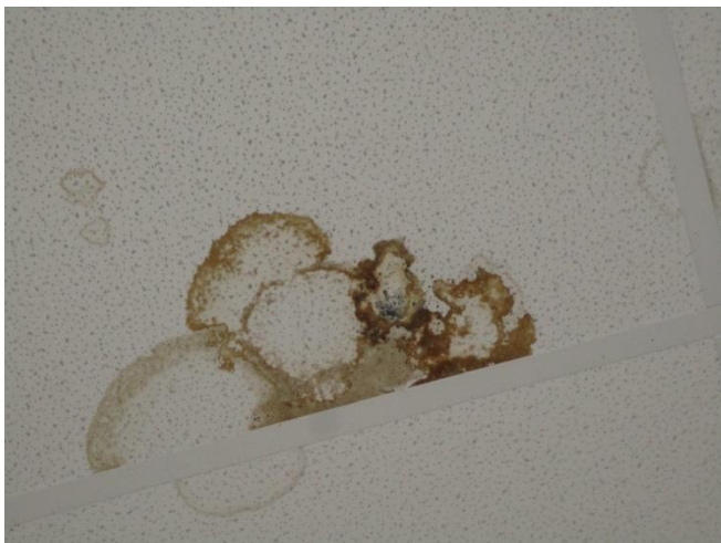
Evidenc of roof leak beneath C1.1
