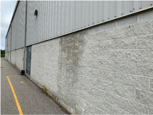
Moisture damage noted on the split-faced concrete block walls.
