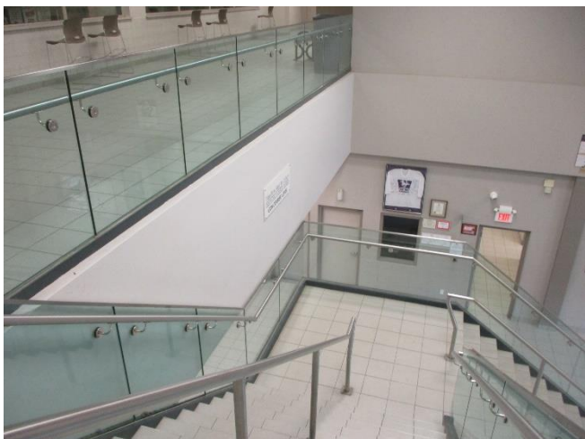
Stairs from the mezzanine to the main lobby were noted in good condition.
